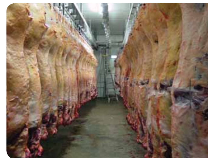
Carcasses in the chiller
